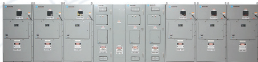
DRAW OUT CIRCUIT BREAKER MTM with (6) 5KV solid state starters
