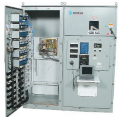
Protective relays and PLC logic
